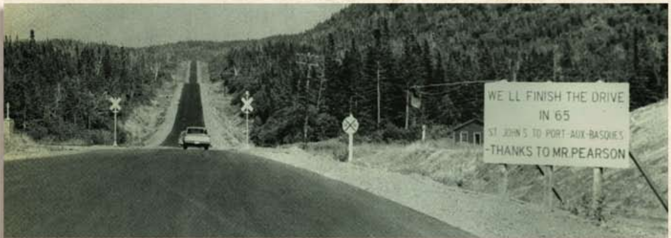
6.54 The Trans-Canada Highway under different phases of construction on the island of Newfoundland, c. 1963-65
